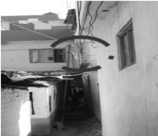
Figure 12: Electric Poles of Pathivara (Source: Author, MSCHS Studio 2017)
